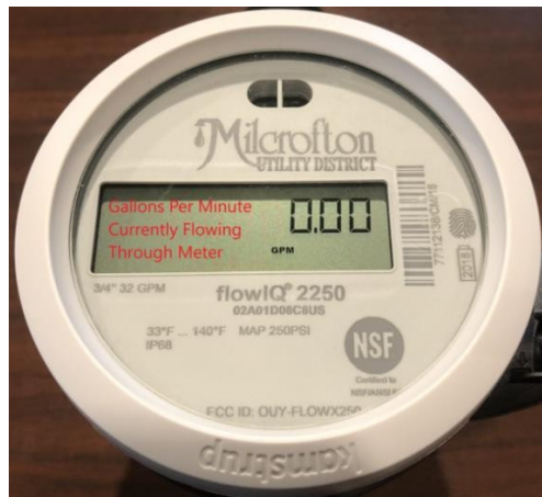
1 of 3 Meter Screens: Total Gallons Metered
